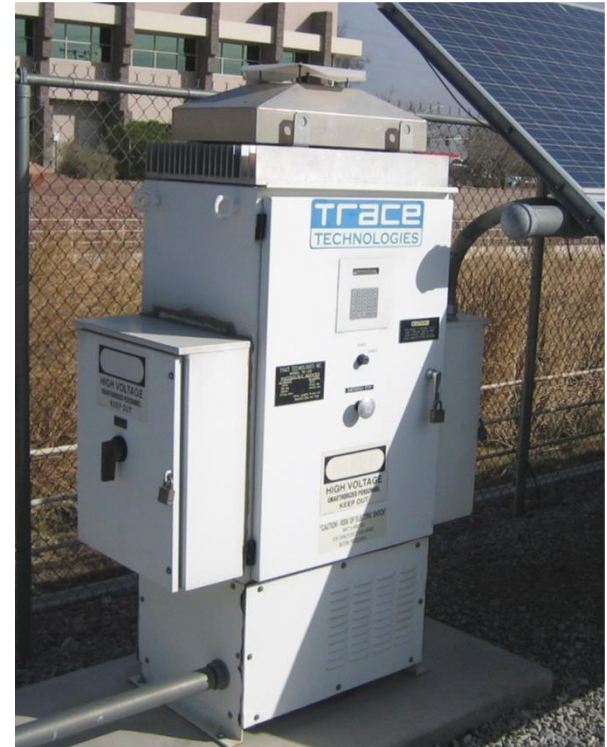
PV Inverter: DC-AC Converter
