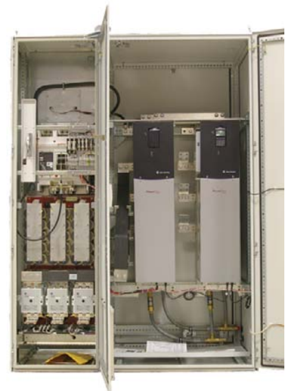
Frame 3B shown (with cabinet doors open)
