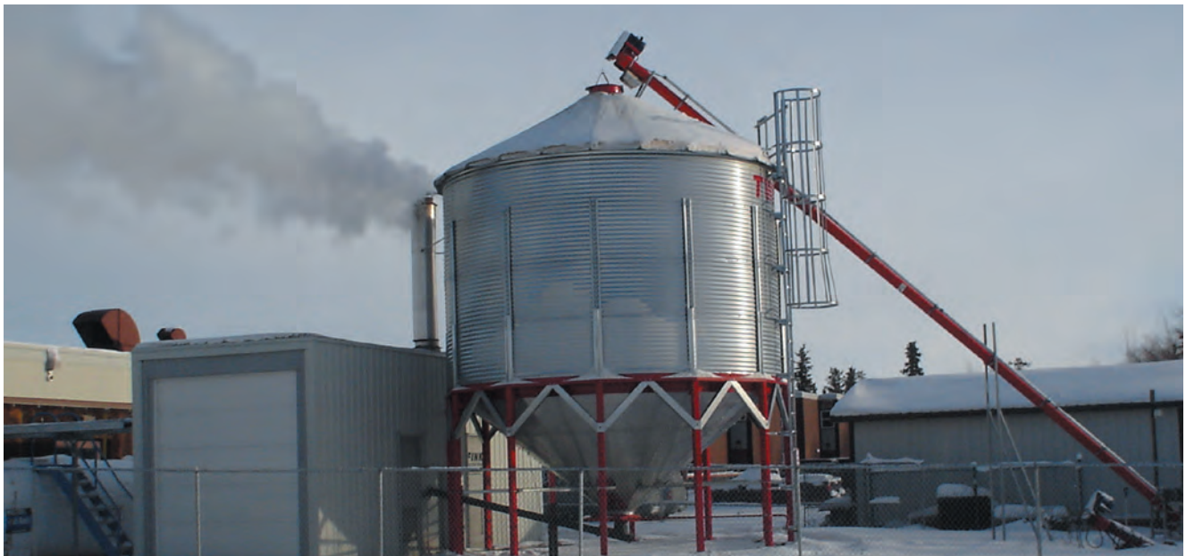
Wood pellet boiler installation at Chief Jimmy Bruneau School in Behchoko, NWT
