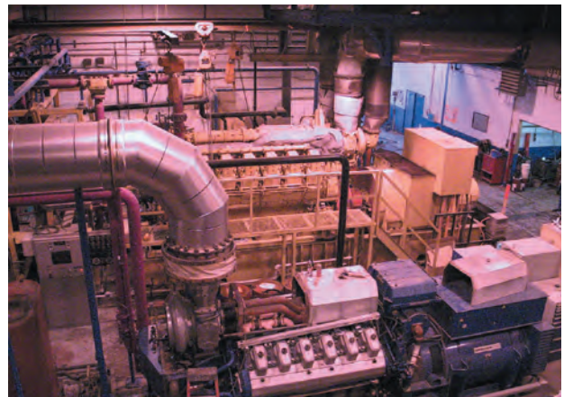
Power Plant, Pond Inlet, Nunavut
