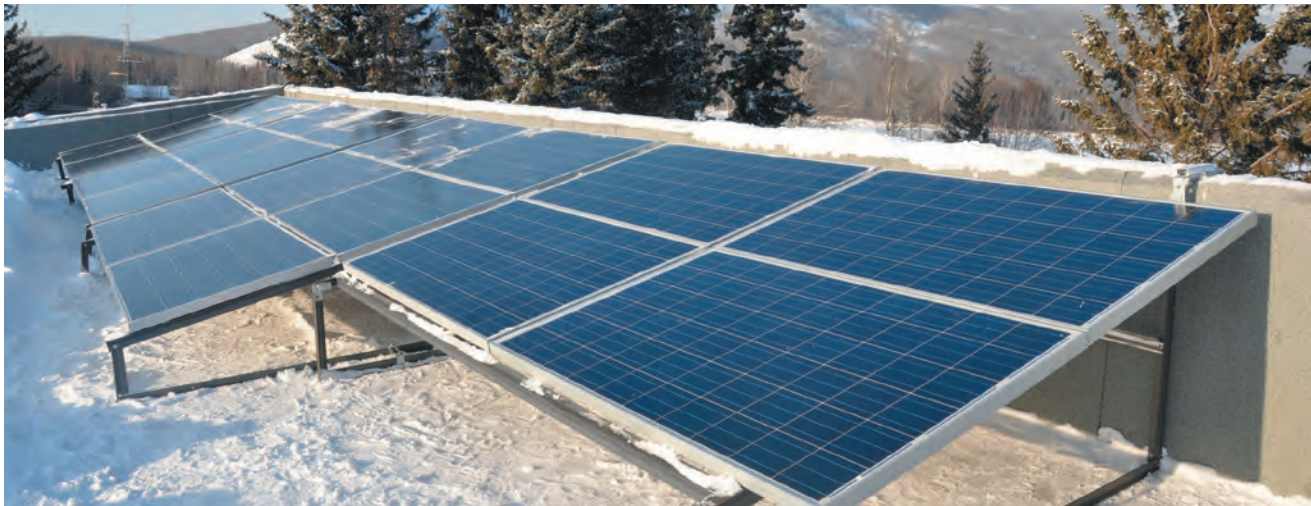
Solar array in Nahanni Butte, NWT
