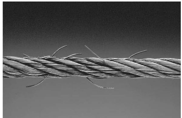
Cable With Broken Wires
