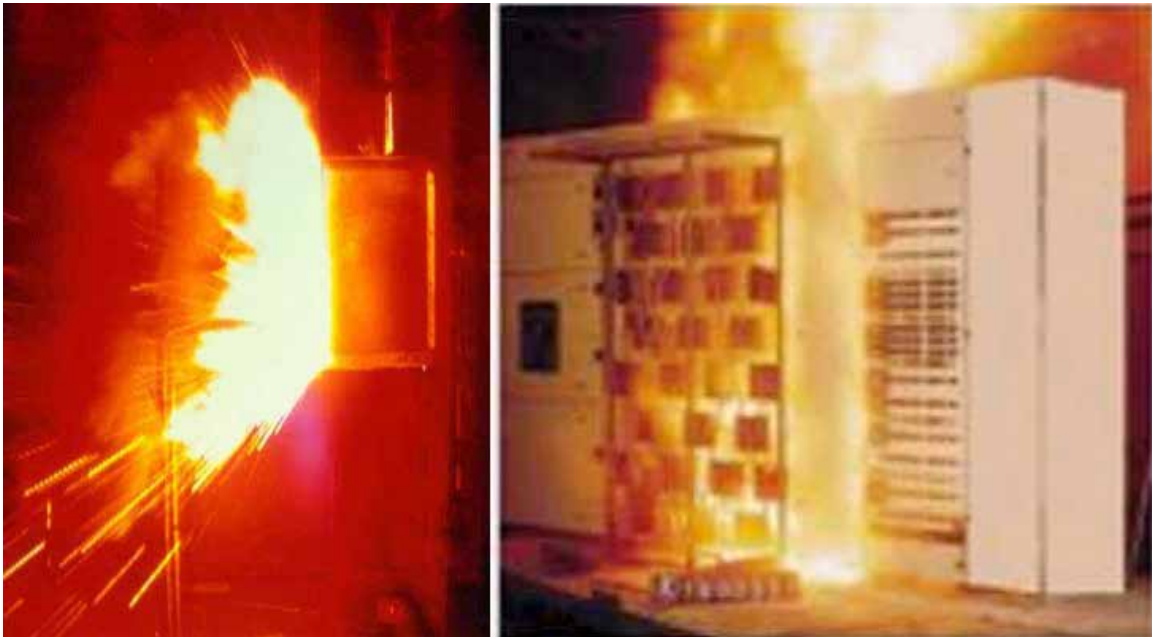
Figure 2.1: (a) Arc Blast in Box; 2 (b) Arcing Fault in an Electrical Panel Board
