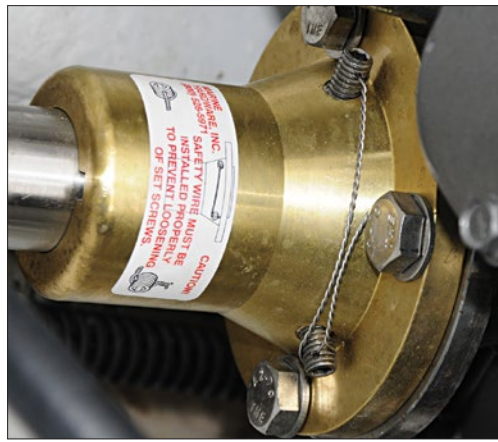
Far left —Grease on this coupling and key was applied to ease installation but will actually prevent full engagement between the shaft and coupling, as it cannot be compressed in the confined coupling bores. Shafts, keys, and couplings may be lightly oiled to prevent binding and ease installation. Left —This brass taper coupling relies on set screws to secure the shaft end nut. Note that the seizing wire is correctly tensioned to rotate the screws clockwise.
