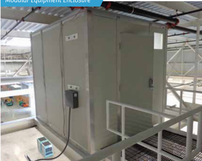
Modular Equipment Enclosure
