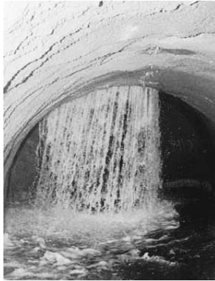
Figure 1.5 Very difficult to seal off by post-injection (photo by courtesy of Oxford Hydrotechnics, UK)
