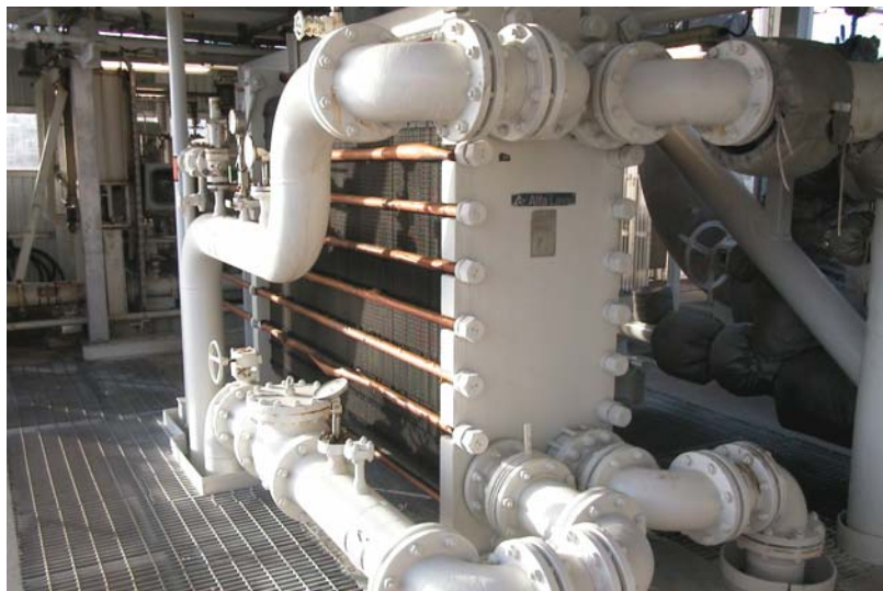
Figure 24 One of the plate heat exchangers in the survey installed in gas compression process
