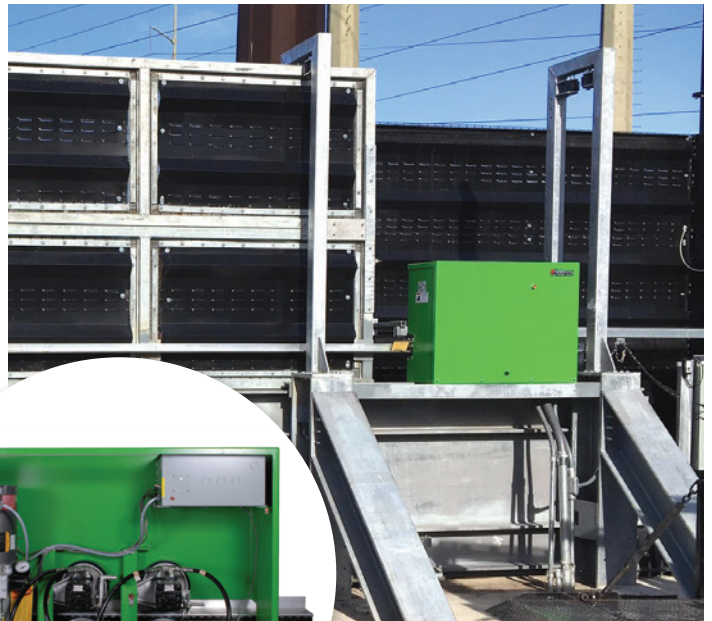
SlideDriver 200 operates crash gate at power substation
