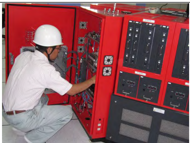
M4F Radar Equipment Room (Transmitter)
