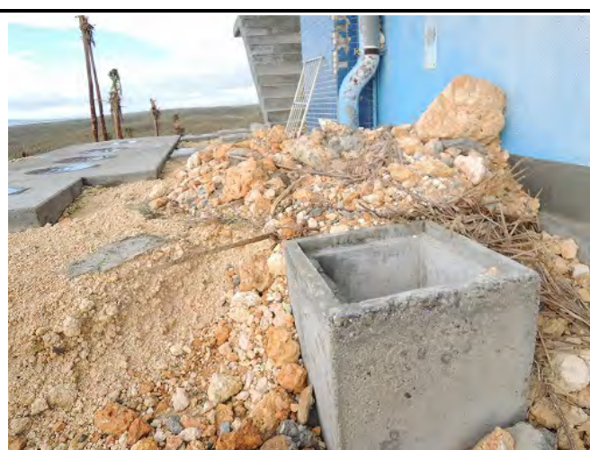
Manhole for Water Discharge (Concrete Cover is damaged)
