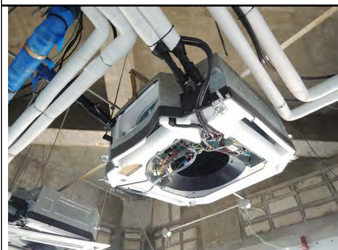
1F Observation Room (Air Conditioning Indoor Unit)
