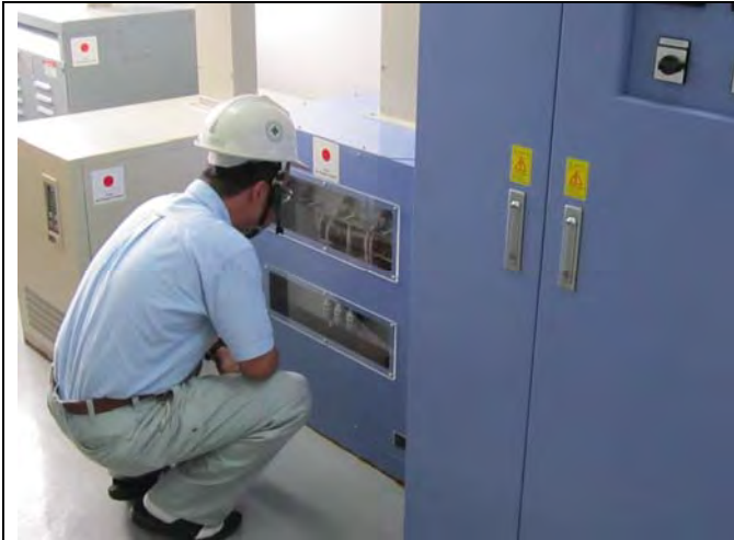
1F Electronic Room (Isolation Transformer and Automatic Voltage Regulator (AVR))
