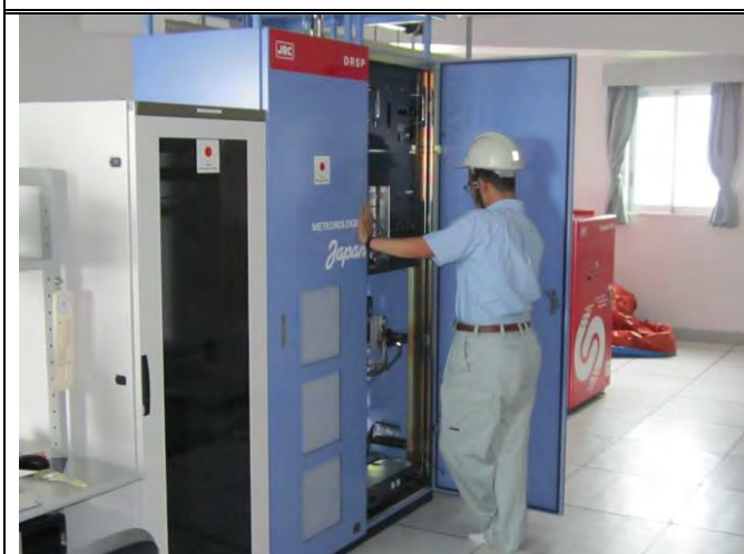
M4F Radar Equipment Room (Digital Receiver and Signal Processor)
