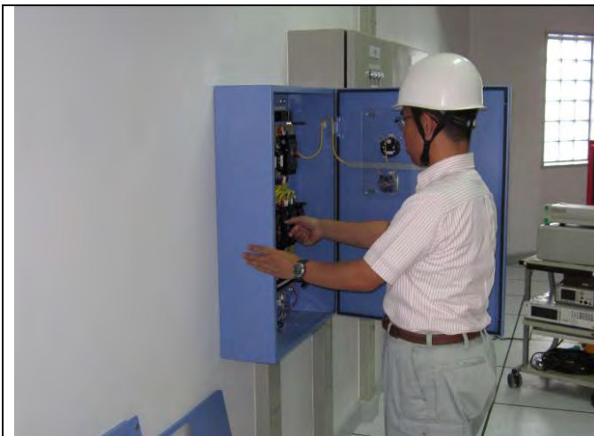
M4F Radar Equipment Room (Distribution Panel for the Radar)
