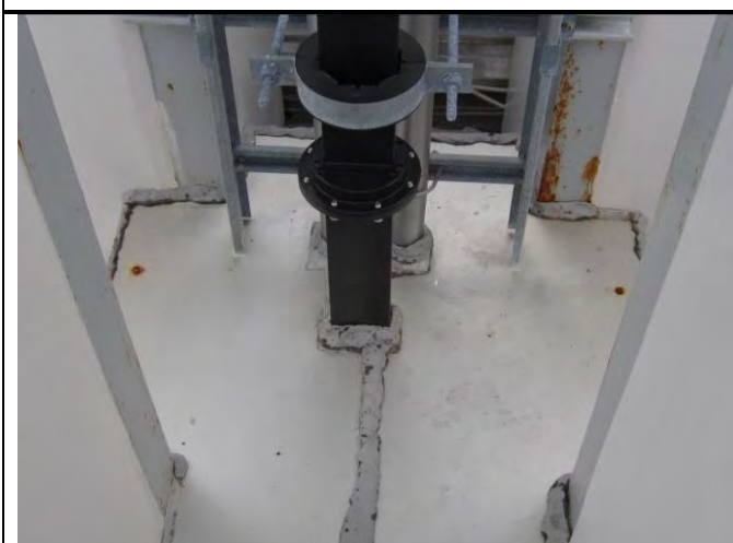
6F Radome Room (Cover of the Cable Duct)
