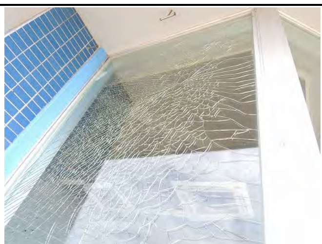
1F Observation Room (Window Glass Broken by Stepping Stones)
