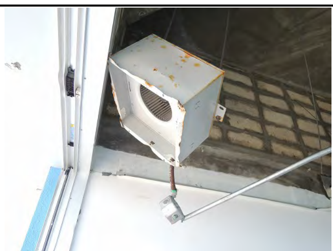
1F Data Analysis Room (Ceiling Exhaust Fan)
