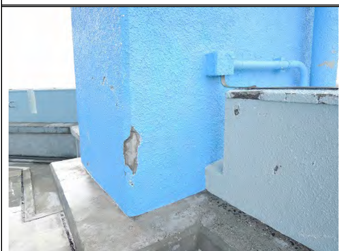
5F Observation Deck (Collision Mark of the Air Conditioning Outdoor Unit)
