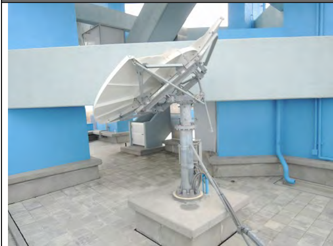
2F Roof (VSAT Antenna)
