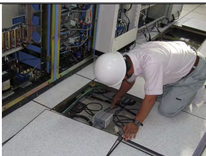
M4F Radar Equipment Room (Under the Access Floor)
