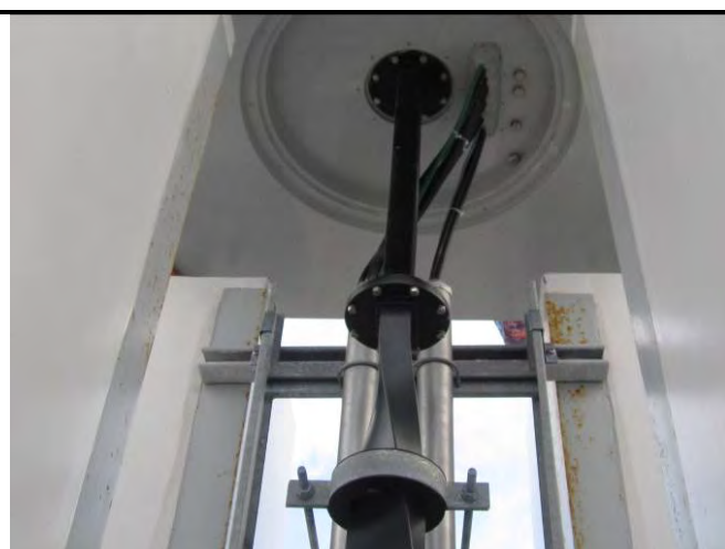
6F Radome Room (Wave-Guide Configuration of the Pedestal Bottom)
