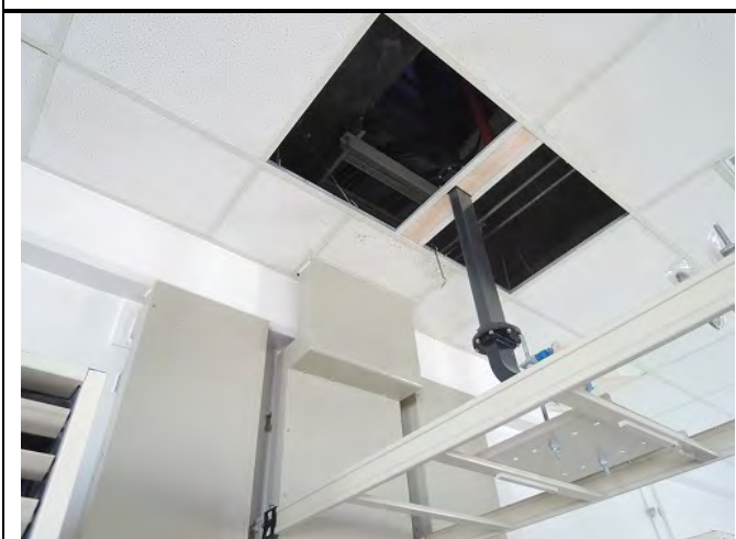
M4F Radar Equipment Room (Ceiling which is located immediately below the 5F Cable Duct)
