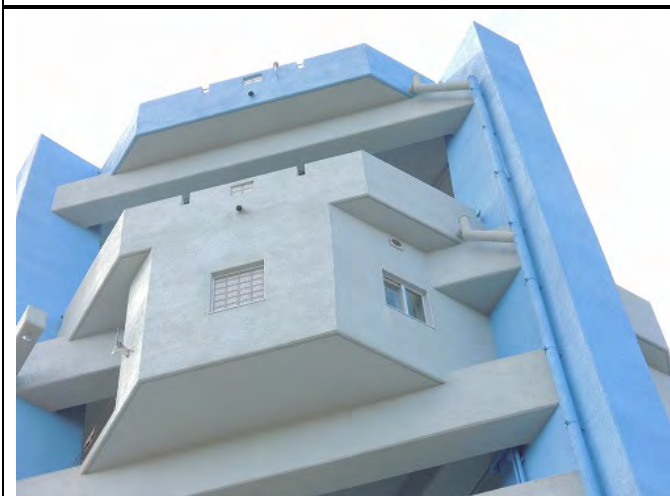
M4F Radar Equipment Room (Southeastern Exterior Wall)
