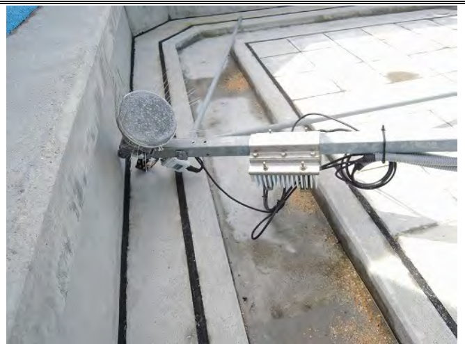
2F Roof (VSAT Antenna)
