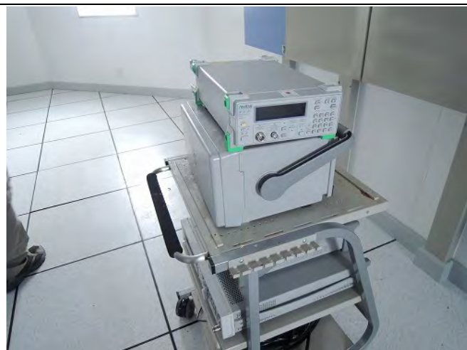
M4F Radar Equipment Room (Measurement Equipment)
