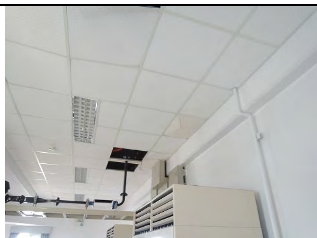
M4F Radar Equipment Room (Ceiling of the 5F Cable Duct Bottom)
