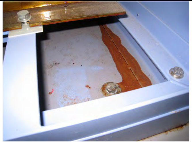
1F Electronic Room (Isolation Transformer)
