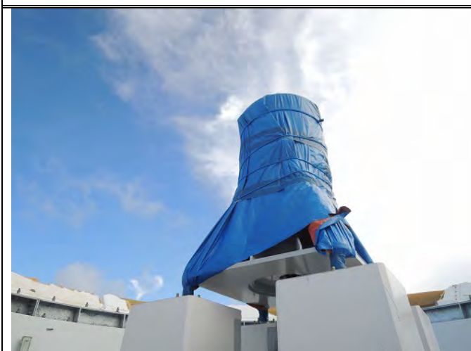
6F Radome Room (Antenna Pedestal)
