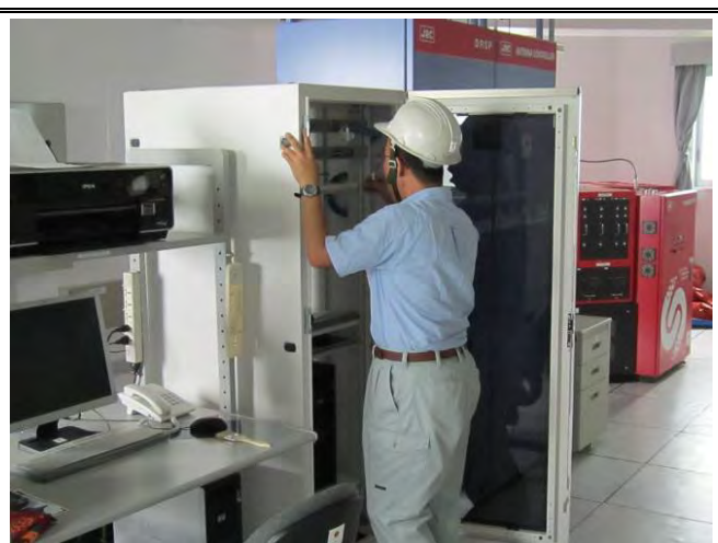
M4F Radar Equipment Room (Data & Protocol Converter)
