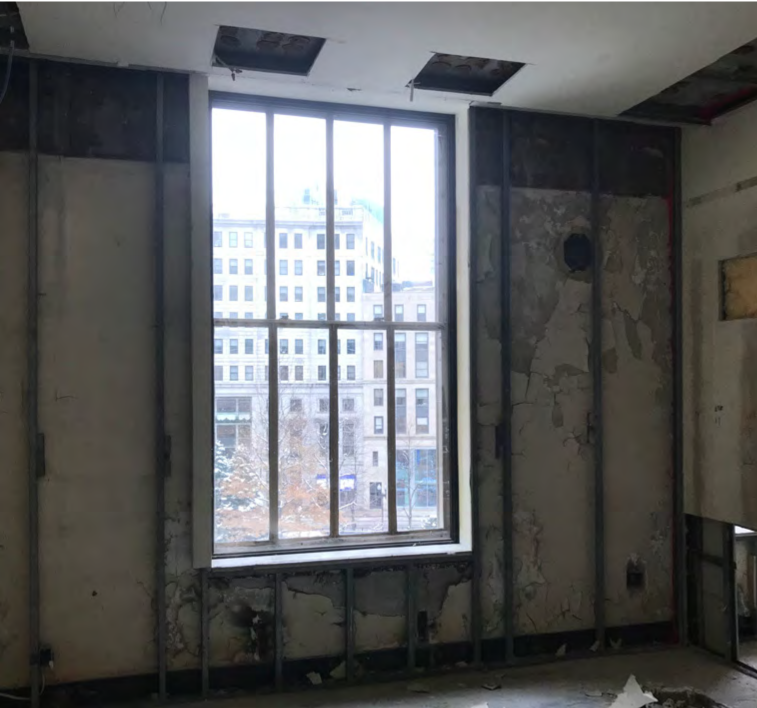
DRYWALL REMOVED DUE TO MOLD AND WATER INFILTRATION
