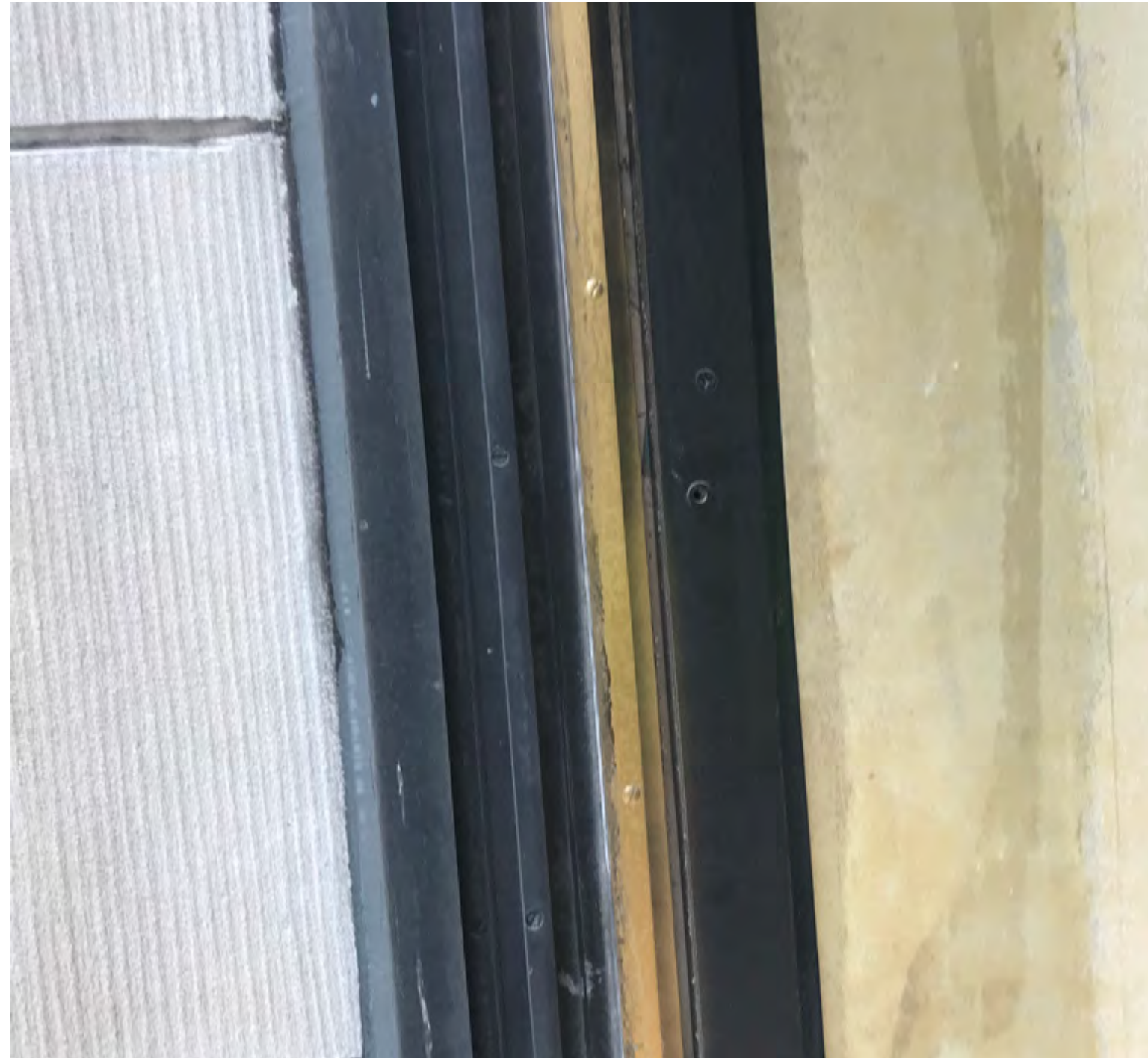
STRAIGHT EDGE OF DOWSIL SEALANT 790/791/795 (LEFT JAMB)
