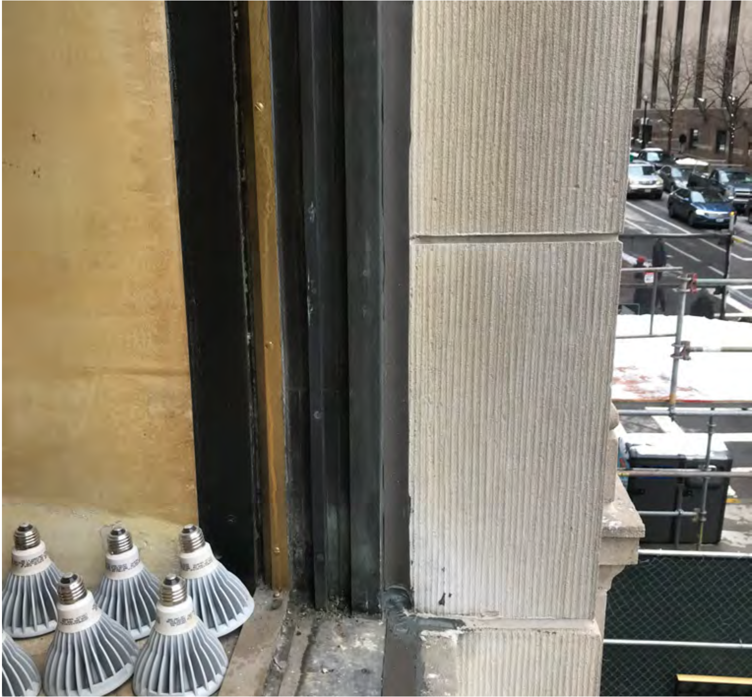
STRAIGHT EDGE OF SEALANT TAPE DOWSIL 123 (RIGHT JAMB)
