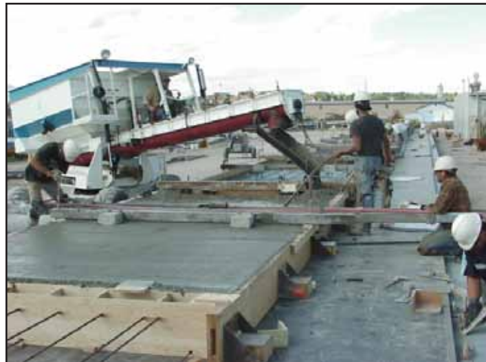
Figure 4.1.o. Placement of concrete backup over insulation. Use of pencil vibrator to consolidate backup mixture.
