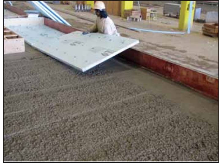
Figure 4.1.d. Placing 2-in.-thick (51 mm) insulation. Insulation is predrilled at 16 in. (406 mm) on center to accept pin-style connectors.
