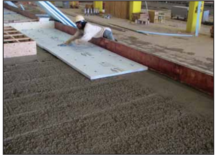
Figure 4.1.e. Placing 2-in.-thick (51 mm) insulation. Insulation can go outer edge to outer edge or can incorporate certain areas of panels that are uninsulated, depending on design criteria required.
