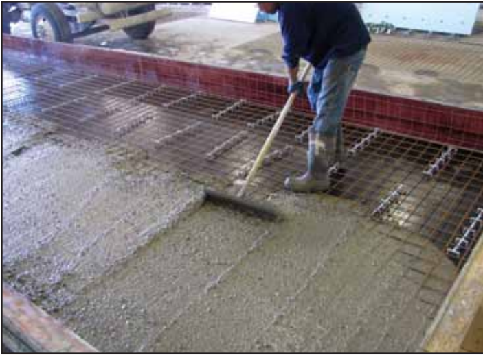
Figure 4.1.b. Concrete being placed as a part of face mixture, raking mixture to cover all surfaces of form. Once placed, concrete will be vibrated with both external and internal units; placement depth is 3 in. (76 mm) for face mixture.
