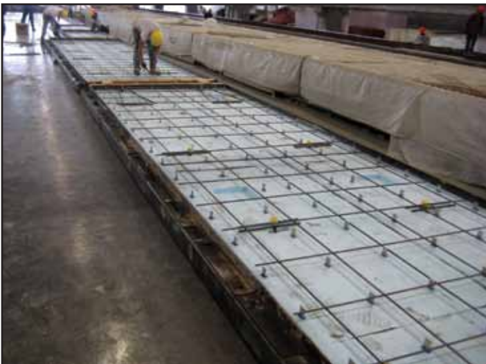
Figure 4.1.i. Pin connectors for composite action. Prestressing strand in place to prestress panel.
