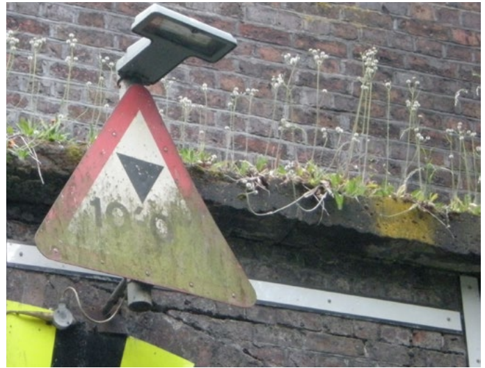
Figure D1: Sign requiring cleaning or like for like replacement
