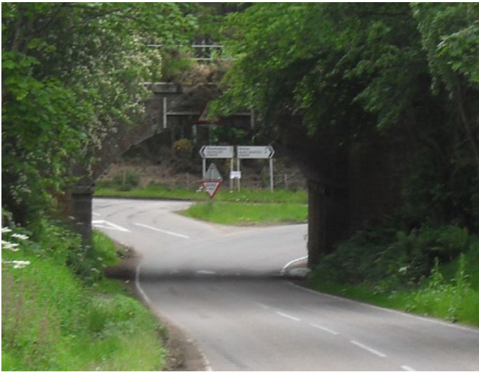
Figure D2: Tree branches overhanging the road obscuring the traffic sign
