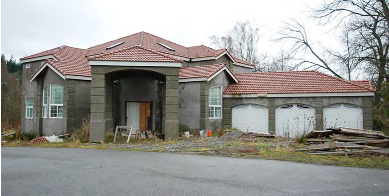
Figure 13.1 Impact of the Great Recession The impact of the Great Recession can be seen in many areas of the economy that impact our daily lives. One of the most visible signs can be seen in the housing market where many homes and other buildings are abandoned, including ones that midway through construction. (Credit: modification of work by A McLin/Flickr Creative Commons)
