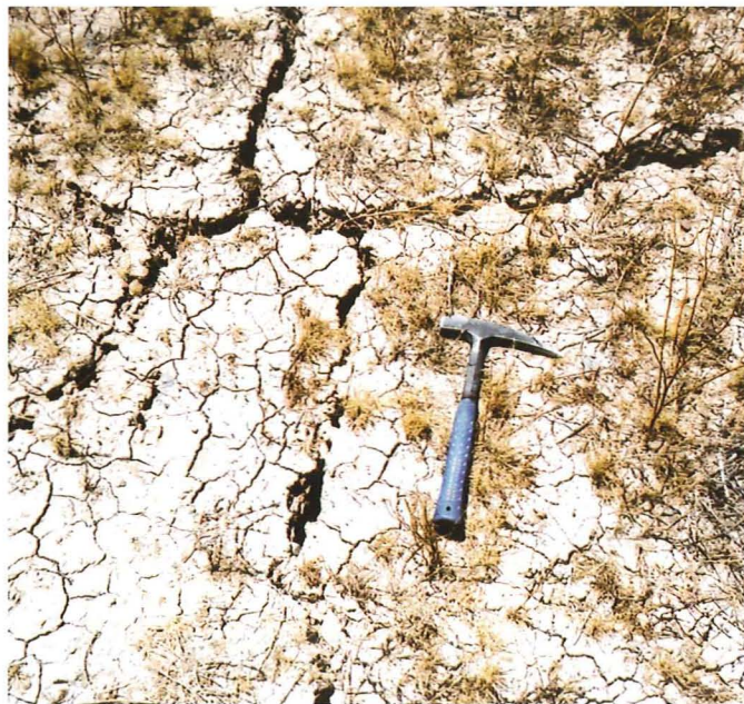
Large cracks in soil indicate extensive drying and shrinking of expansive clay. This type of crack appears during dry seasons. (Photo by Raymond C. Harris)
