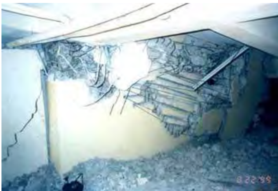
Fig. 19. Heavy damaged shear wall during the earthquake in Turkey 1999
