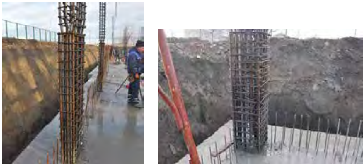
Fig. 35. Problems with clear space between both longitudinal and transverse reinforcement in lapping length of longitudinal bars (the structure was designed according to Eurocodes)
