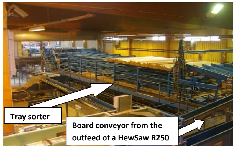
Figure 23: A tray sorter installed at the Havesa Timber sawmill, Hamina, Finland. The sorter can pick up boards and transports them sideways from the conveyor at the end of a HewSaw R250 without elevation of the boards. The tray sorter is an alternative to sling sorters that may cause problems for handling bowed eucalypt boards (source: Washusen 2008).
