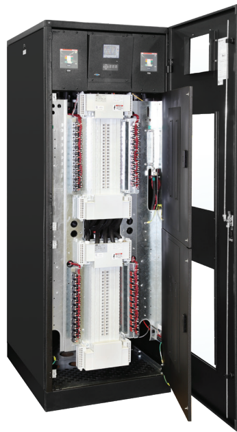
Cyberex® HPP with ABB ProLine panelboards
