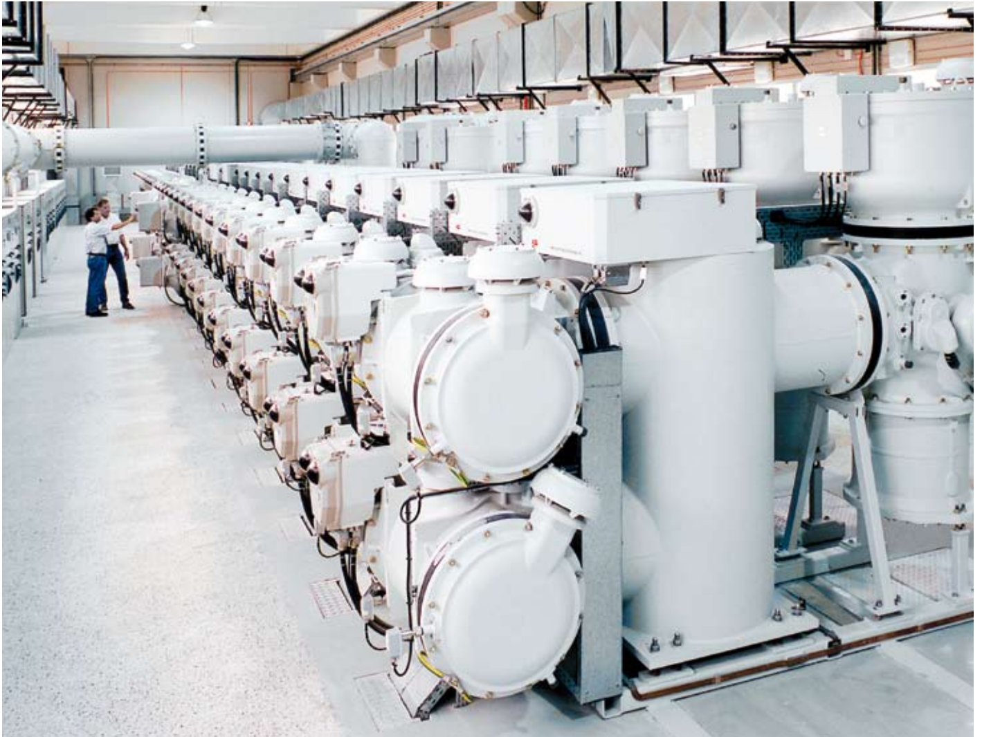
ELK-04 in double busbar arrangement
