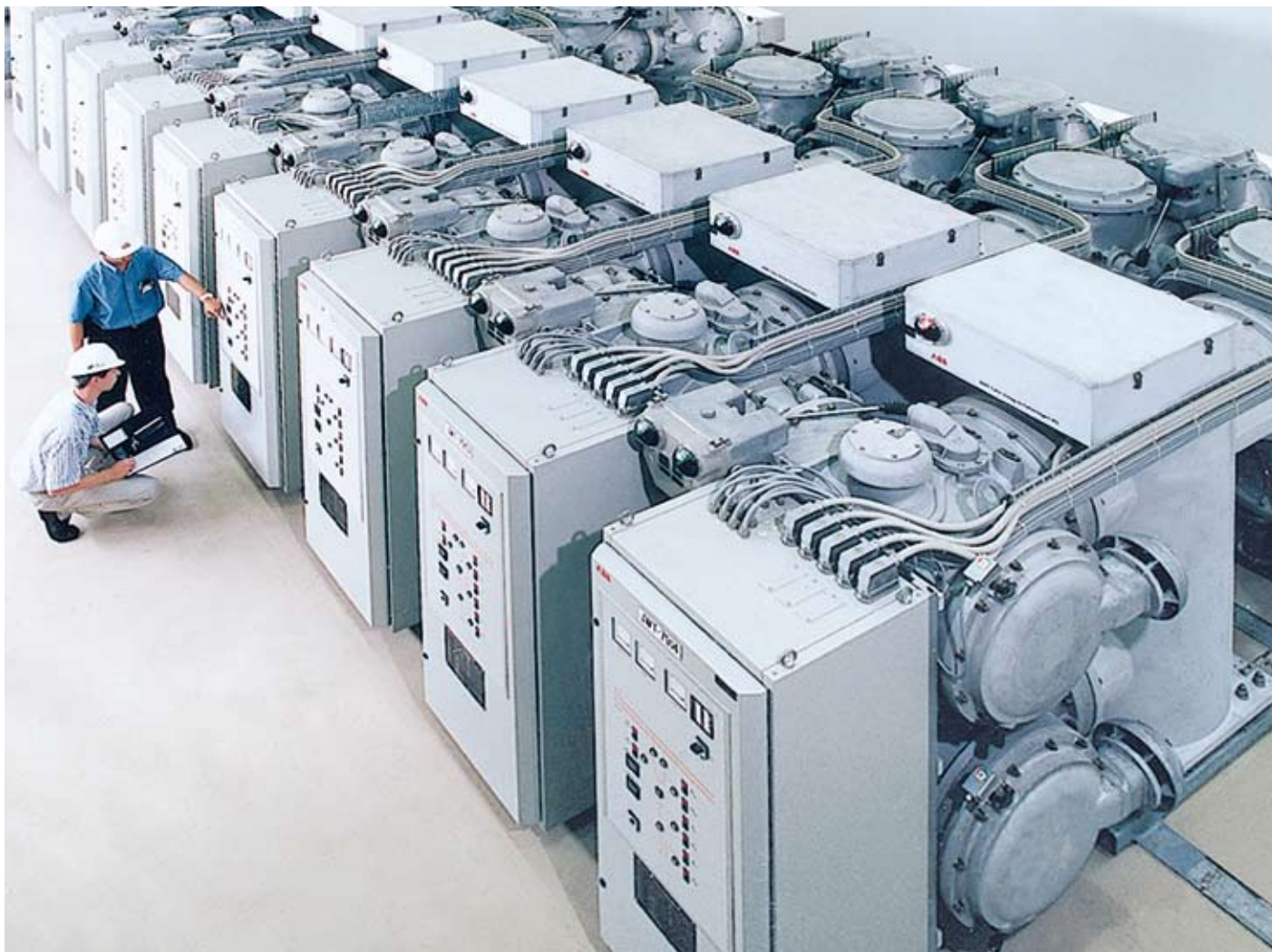
ELK-04 in double bus bar arrangement with integrated local control cabinets
