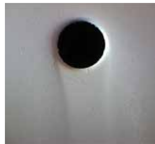
Strong sagging of paint
