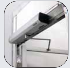
Touchplate-activated Automatic Door
