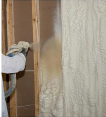
Figure 10: Johns Manville Spray Foam Wall Insulation
