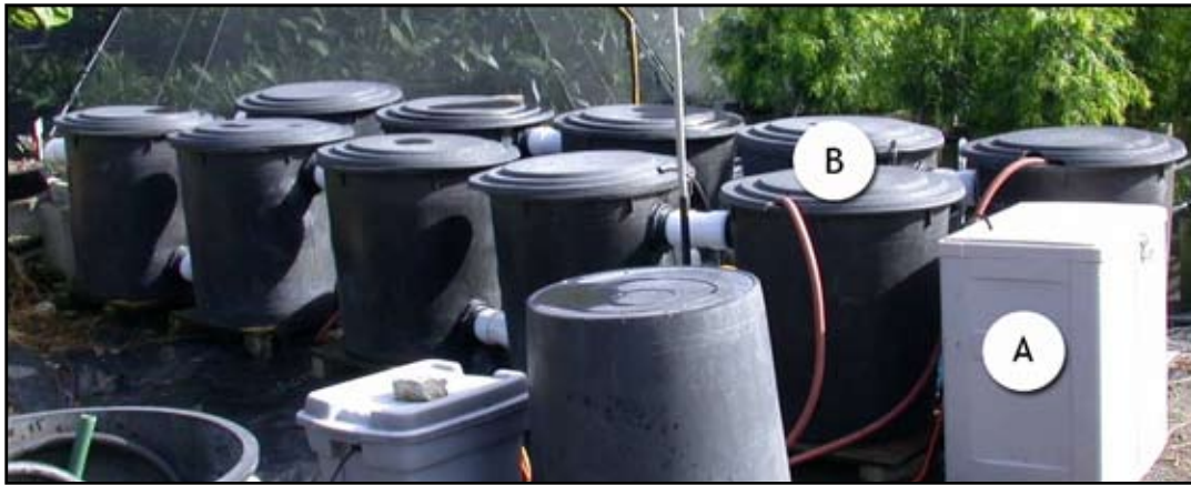
Figure 5. Small-scale bioreactor installed at an ornamental nursery.
