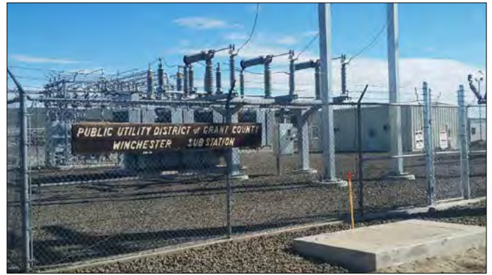
Updated with new equipment that includes a 115kV circuit switcher and 25MVA 115-13.8kV transformer, with new and reused distribution breakers, the Winchester Substation is now ready for future area residential, commercial, and industrial growth.
