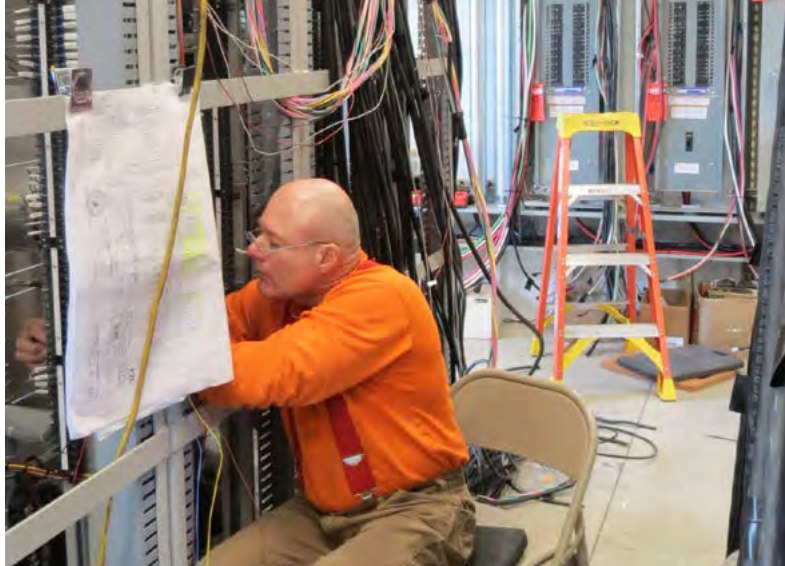
Will Shaw, electrician for Wilson Construction, wires the metering portion of a relay cabinet at the Cloud View Substation, now complete.
