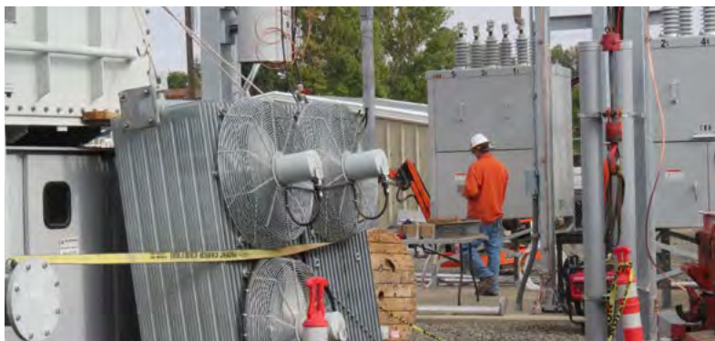
The Central Ephrata Substation was the eighth added to the progressive design build roster after an arc-flash fire destroyed the substation in February 2017. Work was complete by late October.
