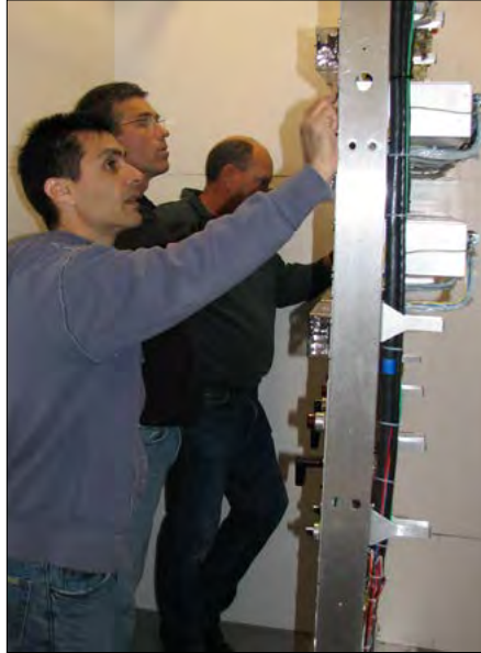
Cowlitz PUD Relay Technicians Joe Furer, Ron Johnson, and Dale Axon work in the Columbia Way Substation.
