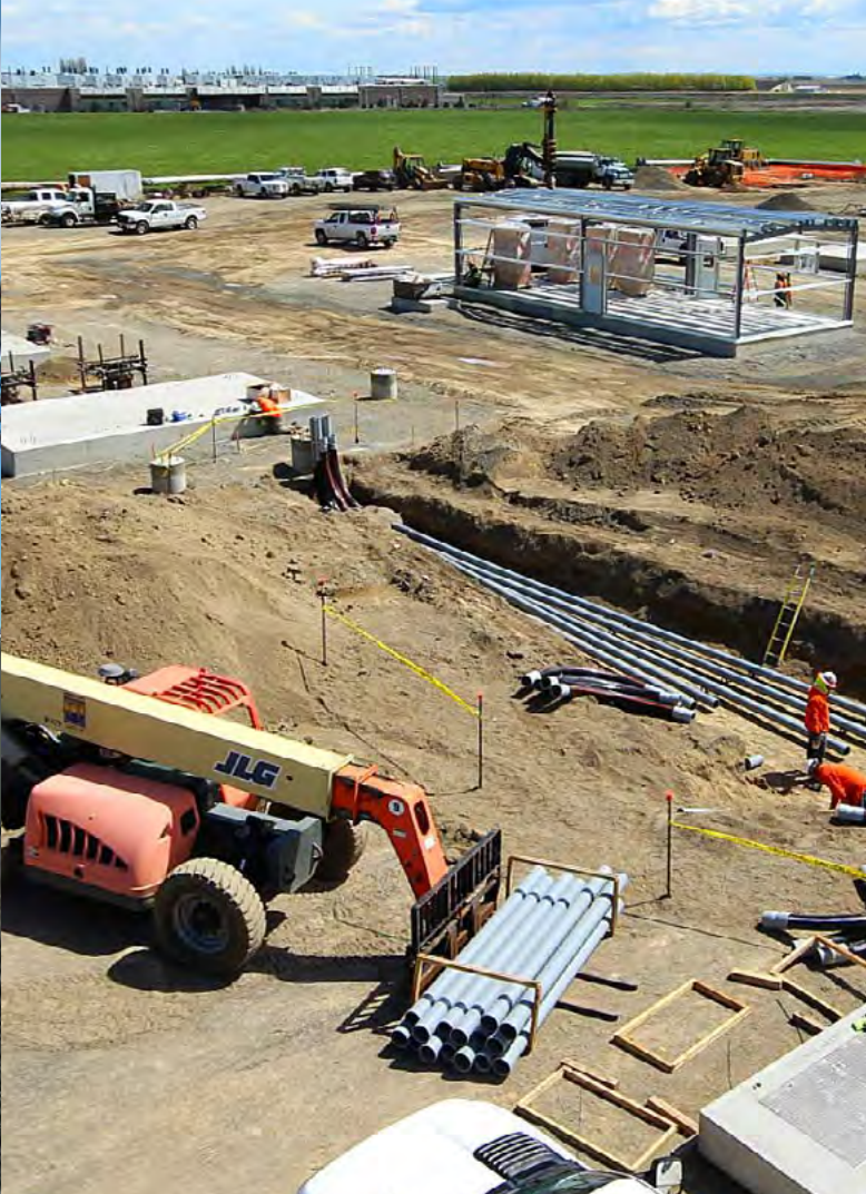
Early construction at Cloud View substation shows crew at work as one of the data centers that is driving the need for system expansion operates in the background.
