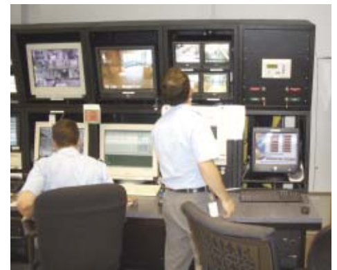
Security guards monitor CyberStation alarms 24/7/365
