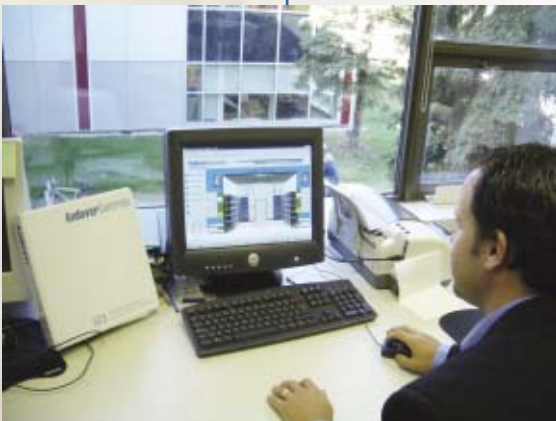
Continuum workstation operator monitors cold room parameters
