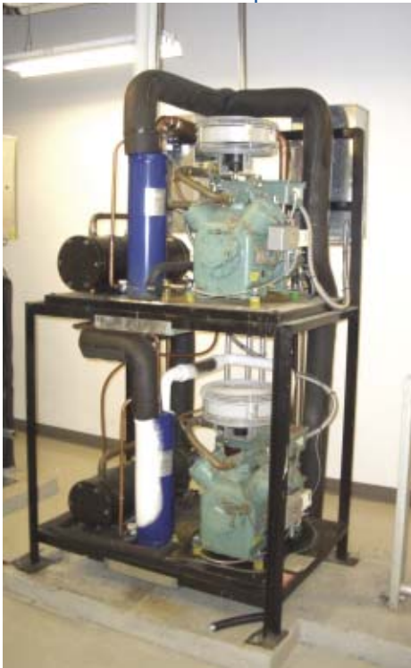
Redundant compressors for one of Héma-Québec's cold rooms
