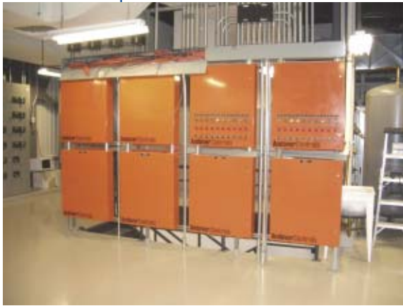
Redundant Continuum controllers for cold room control
