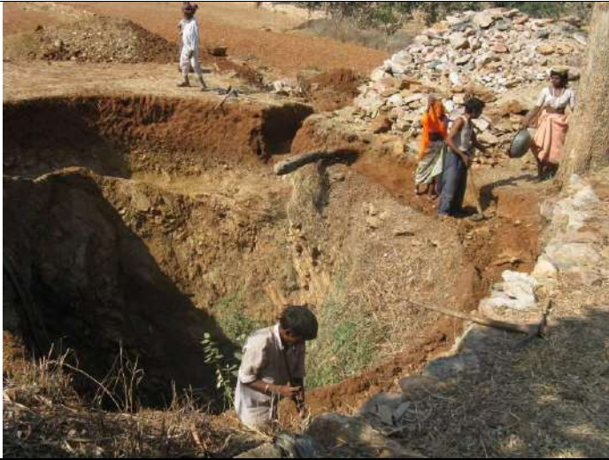
Community participation and gender equity maintained during well lining construction at Sawna
