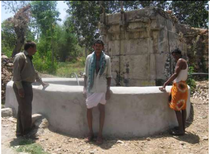
Well owners standing aside to the newly developed well lining at Ramela
