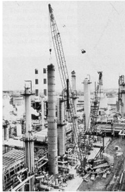
Figure 1-4: Construction of a Benzene Plant in Lima, Ohio (courtesy of Manitowoc Company, Inc.)
