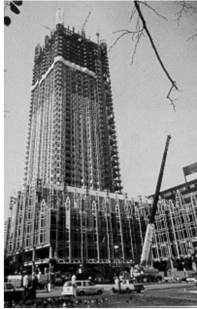
Figure 1-3: Construction of the PPG Building in Pittsburgh, Pennsylvania (courtesy of PPG Industries, Inc.)
