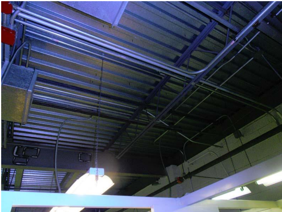
58. Photograph of the underside of the metal deck substrate on Roof Area F. Please note the mechanical fasteners used to mechanically fasten the base layer of insulation. Also please note the electrical conduit running along the underside of the metal deck substrate. The roofing contractor must be cognizant of the conduit running along the underside of the metal deck substrate during roof replacement.
