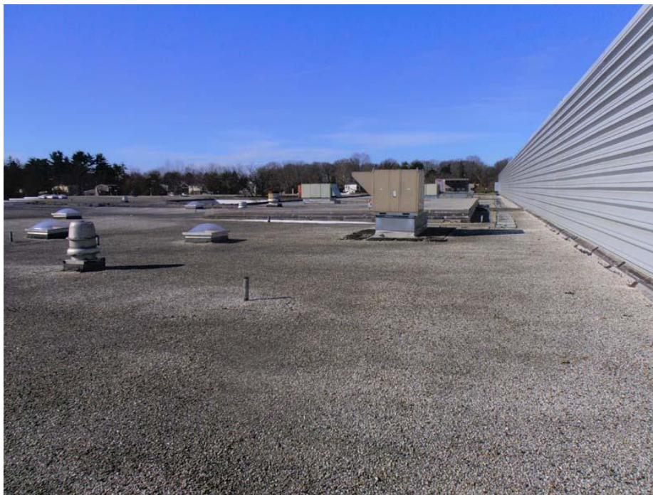
20. An additional overall photograph of Roof Area C. Leaks are reported below this roof area within the field of the roof. Tarps, hoses and buckets are utilized to catch the leaks.
