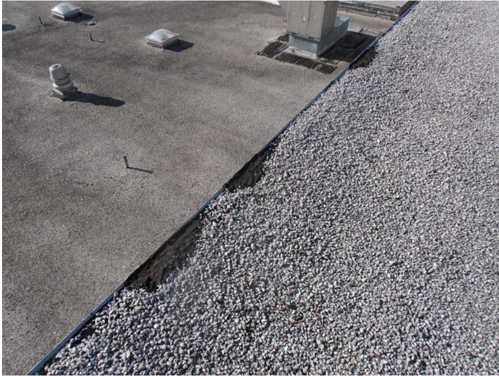
57. Photograph taken on Roof Area I showing some of the repairs to the perimeter with roof cement.
