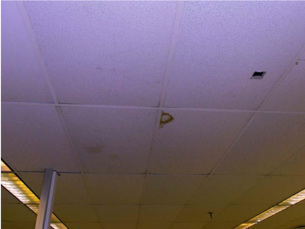
61. Damaged ceiling tiles below Roof Area D.
