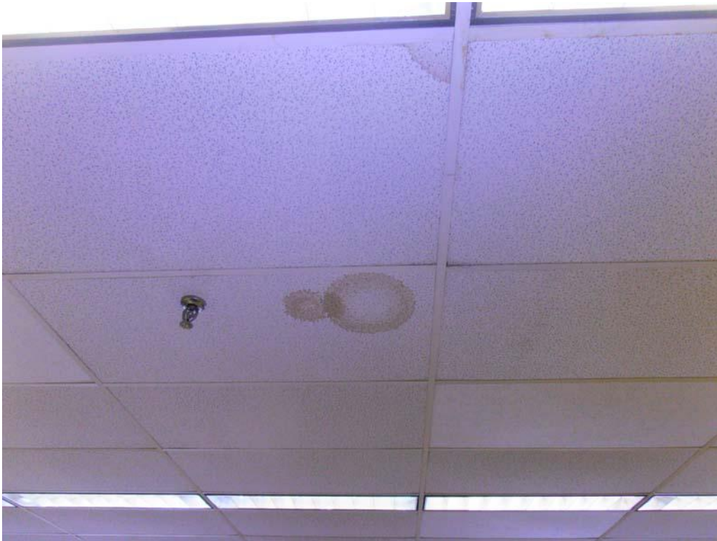
59. Damaged ceiling tiles from leakage below Roof Area D.
