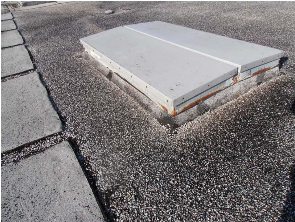
49. Photograph of one of the smoke hatches on Roof Area G. Please note the base flashing at corners and overlapping seams have been repaired with roof cement.
