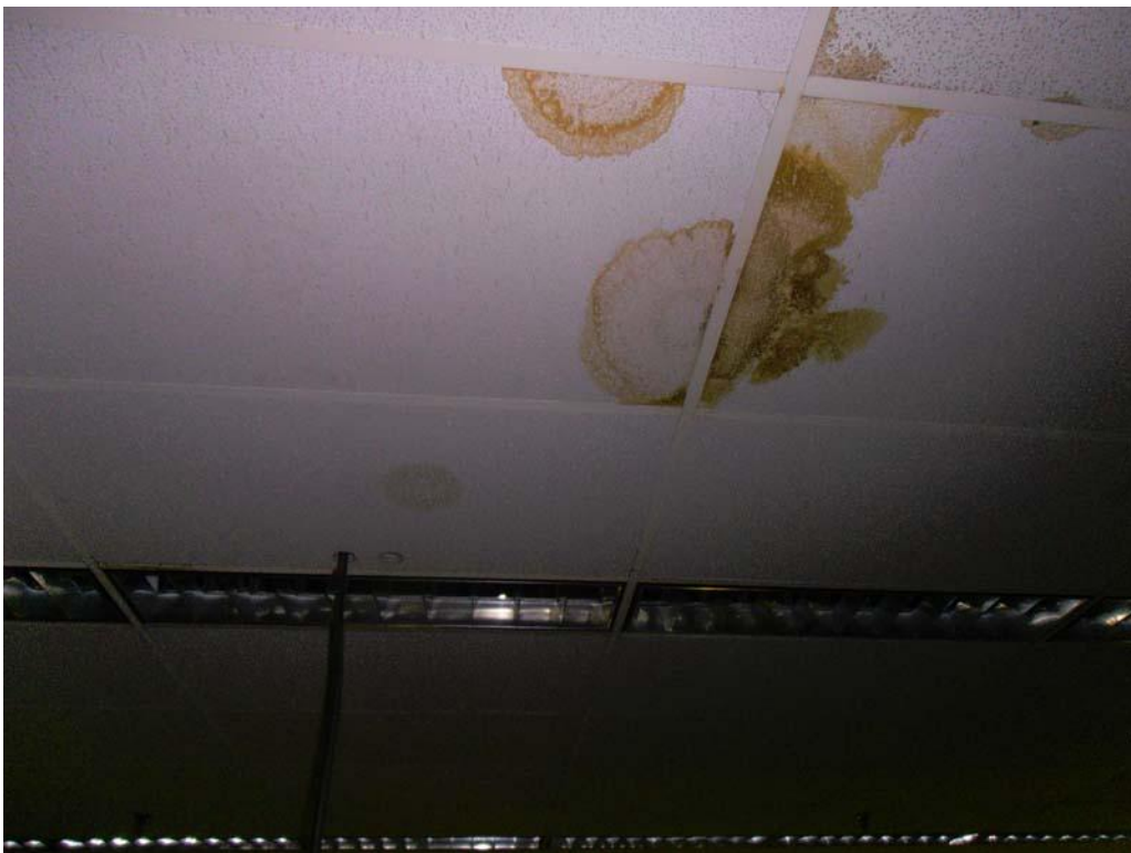
60. More damaged ceiling tiles below Roof Area D. Note the hose extending through the ceiling tile to drain moisture.
