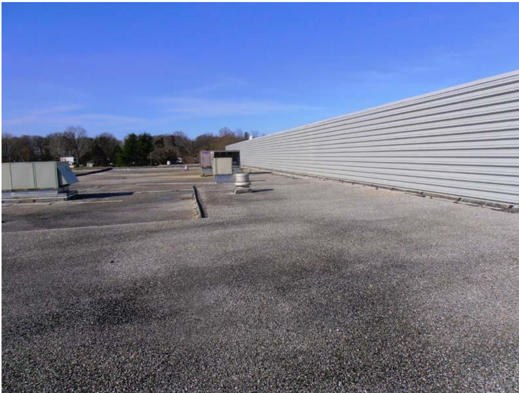
28. An additional overall photograph of Roof Area D1. Roof Area D1 incorporates the same roof assembly as Roof Area A; however, the deck substrate is concrete and therefore the base layer of flat insulation was set in asphalt in lieu of mechanical fastening.
