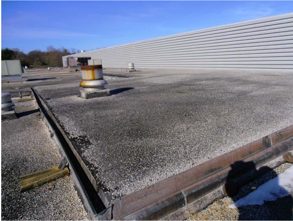
27. Overall photograph of the aggregate surfaced built-up roofing system over Roof Area D1. Roof Area D1 incorporates good slope, sloping in one direction to hanging gutters with downspouts.
