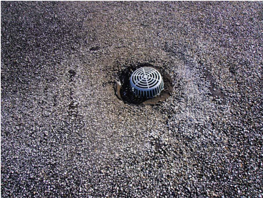
33. Photograph of asphalt repairs where the built-up membrane extends under the drain clamping ring on Roof Area E.
