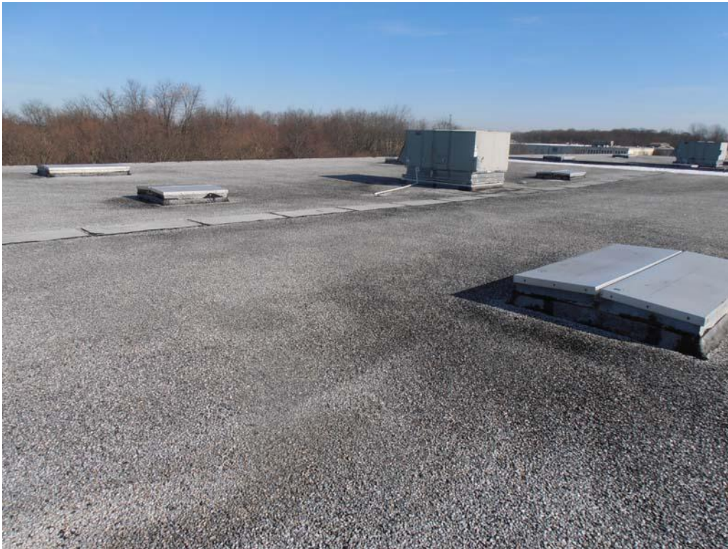
51. Overall photograph of Roof Area H. This roof incorporates excellent slope built into the structure. However, as with the other roof areas, the roofing membrane has dried out over time.
