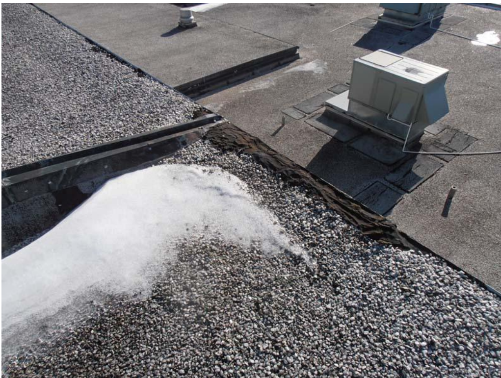
50. Photograph of roof cement repairs to the perimeter at Roof Area G. The stripping at the perimeter became brittle, drying out, and roof cement repairs were required in this area.
