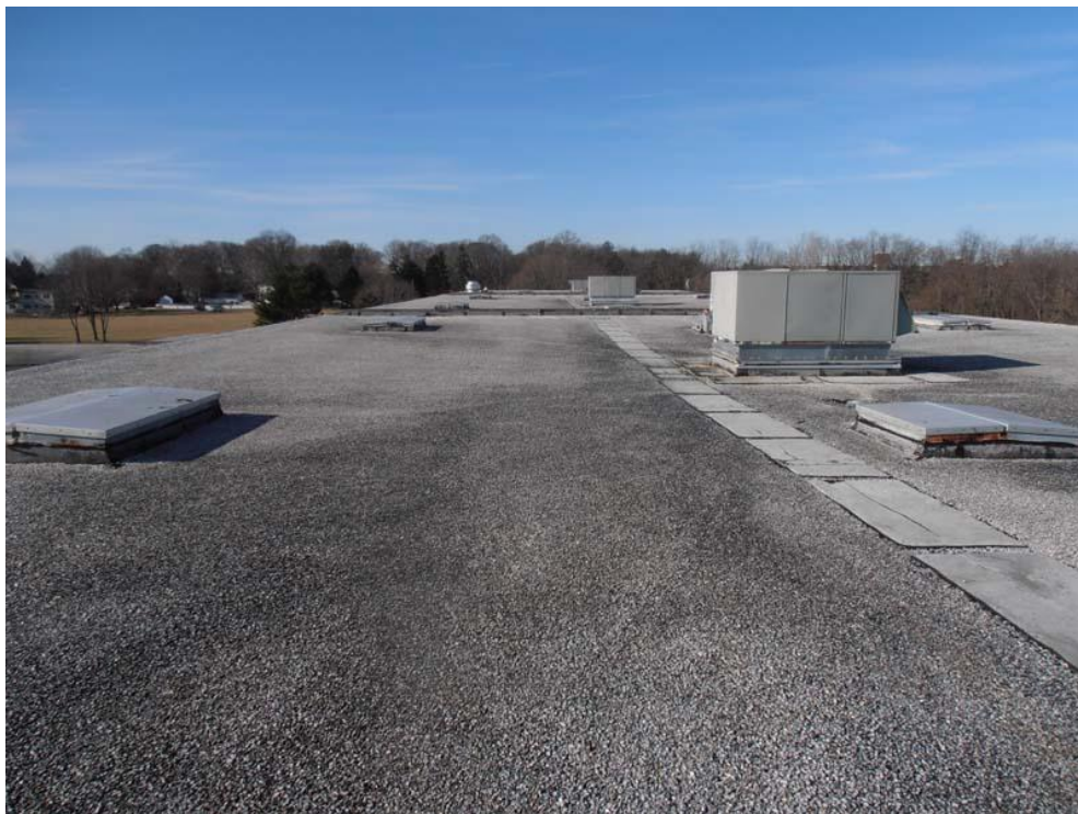
52. An additional overall photograph of Roof Area H. This roof area incorporates similar deficiencies at equipment as other areas with overlapping seams and corners of equipment curbs repaired with roof cement.
