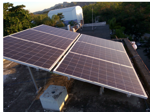
Figure 2: Six photovoltaic models installed of 1,5 kWp
