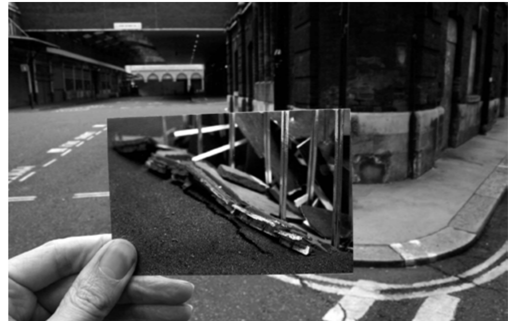
1. Subsidence in Smithfield. Image from Sophie Warren & Jonathan Mosley, (2011) 'Beyond Utopia' Berlin/Los Angeles: Errant Bodies Press.
