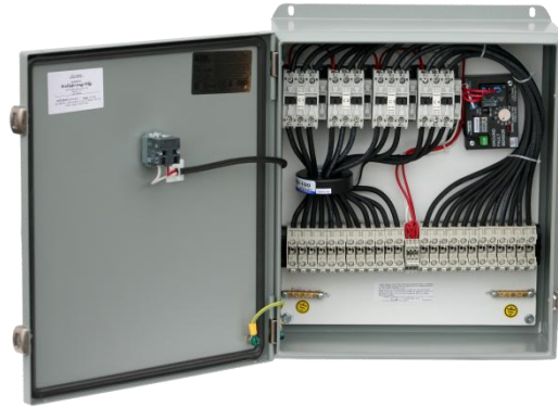
Contactor Panel with GFEP
