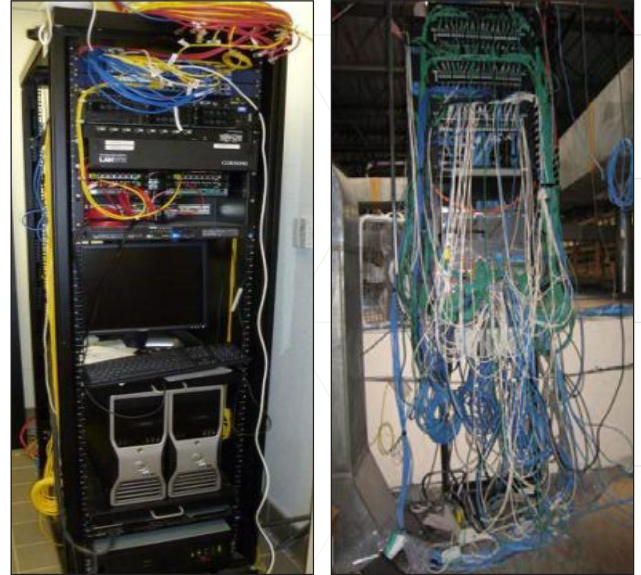
Figure 2. Poor Industrial Network Installation Can Generate Unacceptable Downtime Risks
