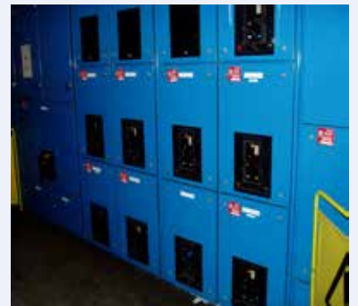
Obsolete Merlin Gerin Selpact ACBs
