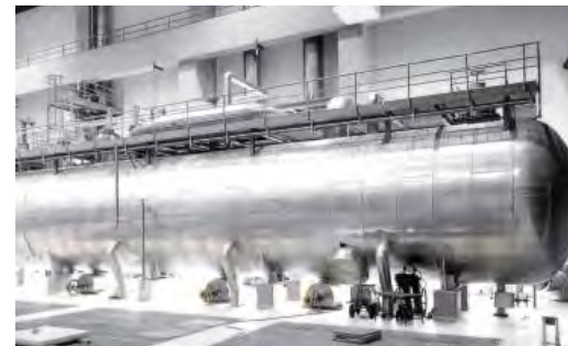
Deaerator / Feedwater Tank
