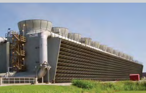
Crossflow Cooling Tower USA
