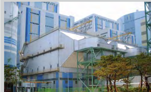
2 x 500 MW ESP Project Korea
