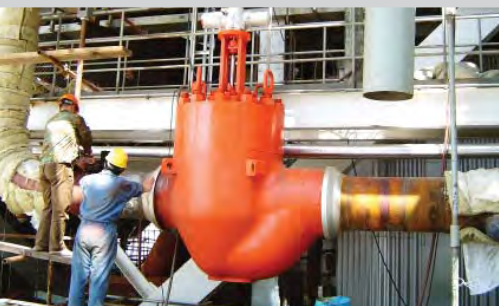
Gaozi Power Plant China
