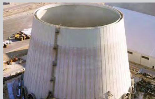
Forced Draft Cooling Tower Saudi Arabia
