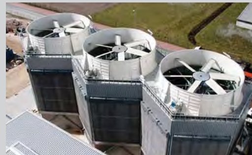
Hexacool Air-cooled Condenser Germany
