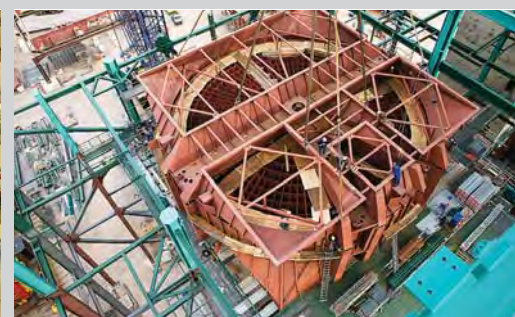
600 MW Air Preheater Project Germany
