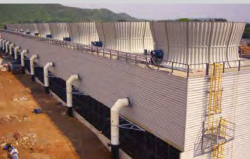
Counterflow Cooling Tower Mexico
