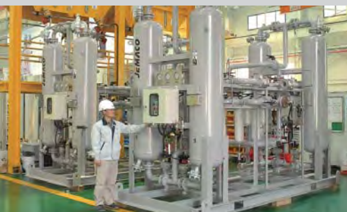
Sidi Krir and El Attf Combined Cycle Power Plant Egypt
