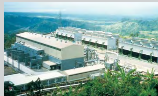
Counterflow Cooling Tower Philippines
