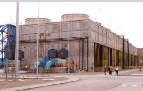
Counterflow Cooling Tower Spain
