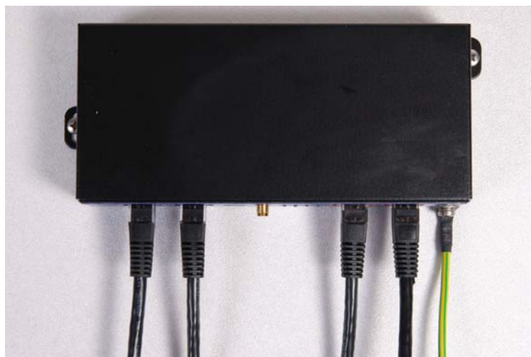
Figure 14 PTP-SYNC mounted on wall
