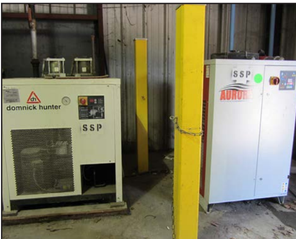
DOMINICK HUNTER & AURORA AIR DRYERS & AIR HOLDING TANK
