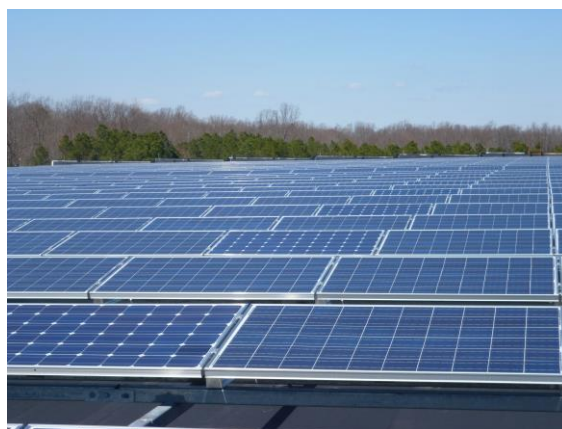
Sharp 240 watt Modules on Rooftop System
