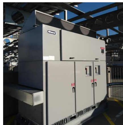
Advanced Energy PVP 260kW Inverter
