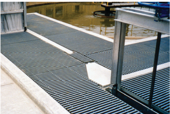
Low maintenance fiberglass grating provides trouble free operations for the covers and walkways in the Lakewood, Colorado Wastewater Treatment Plant Headworks. I-6000 1-1/2" was used.
