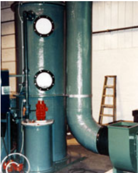
Figure 3. This compact packed tower scrubbing system relies on two very different thermoplastic pumps: a flexible liner peristaltic type rotary pump to meter 50% NaOH on demand to the vertical in-tank circulating pump, which provides a continuous flow of 5% NaOH scrubbing fluid to the tower.
