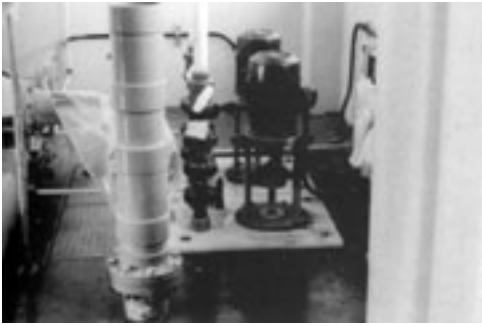
Figure 2. Two Vanton polypropylene sump pumps handling caustic soda and chlorine solutions.
