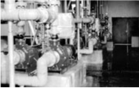
Figure 1. Overview of compact odour-scrubbing installation showing the six Vanton ANSI end-suction polypropylene pumps handling acid and alkaline solutions over the pH range from 3 to 12 at 650 gpm against a 38' TDH.
