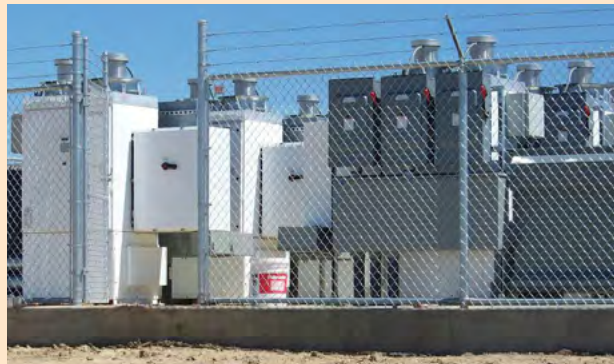
Figure 57. Utility-scale inverters use higher DC input and AC output voltages to reduce losses, and the size and costs of the conductors and switchgear required.
