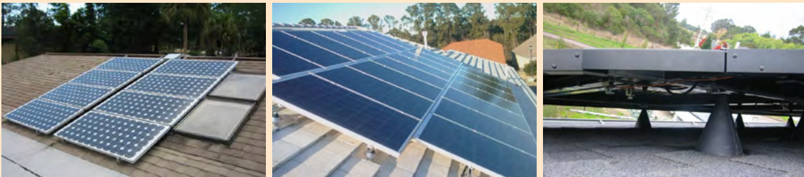
Figure 21. Standoff mounts are the most common way PV arrays are attached to sloped rooftops.
