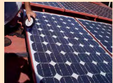
Less obvious fractured glass
