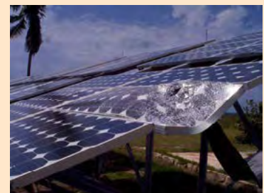
Obvious impact damage
