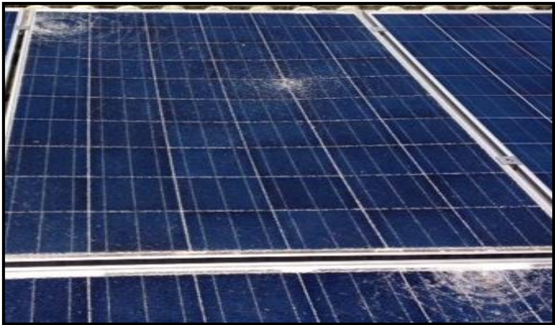
Figure 46: Hail damaged PV module (Source: (Gold Coast Solar Power Solutions, 2014))
