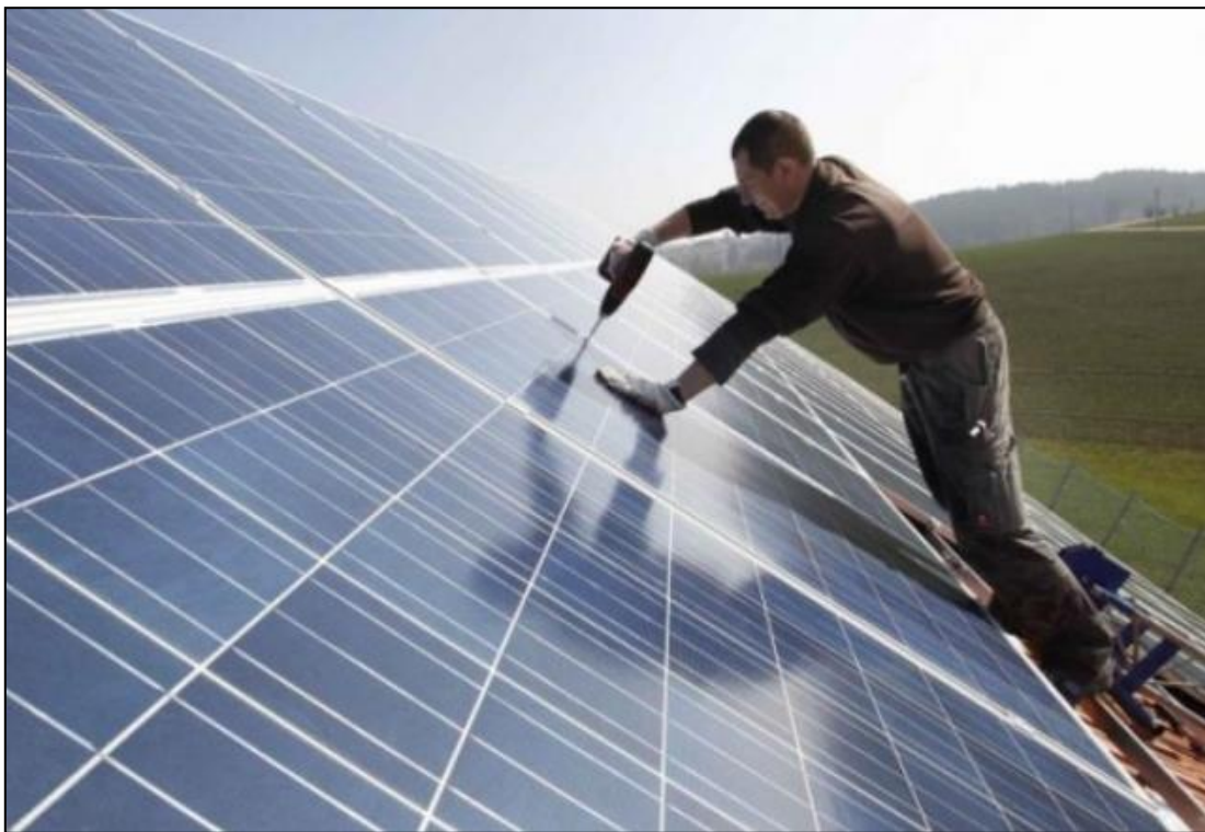
Figure 40: Installer leaning on PV module may cause module to crack (source: (Roest, 3 quality issues in solar panels, 2013))
