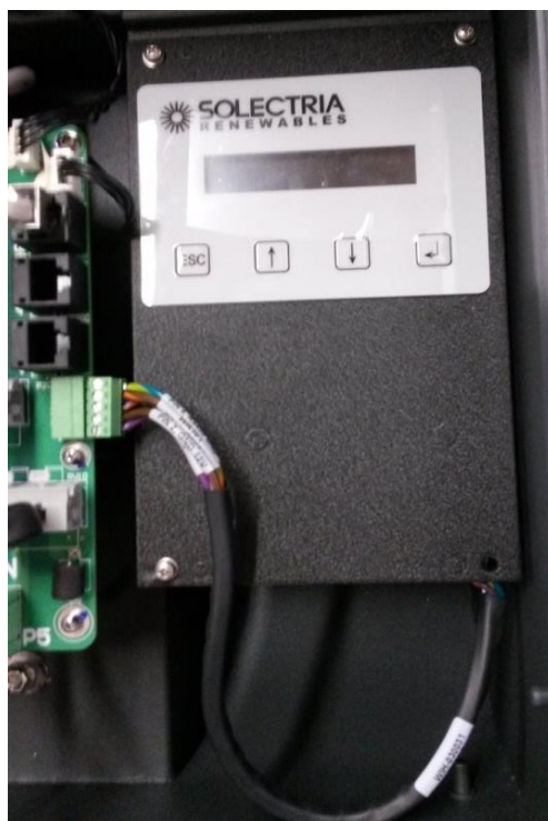
Figure 7.3 SolrenView Gateway Installed into Subcombiner
