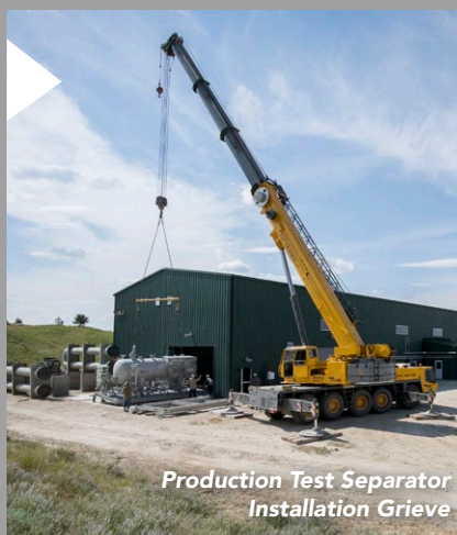
High Pressure Compression Installation Grieve
