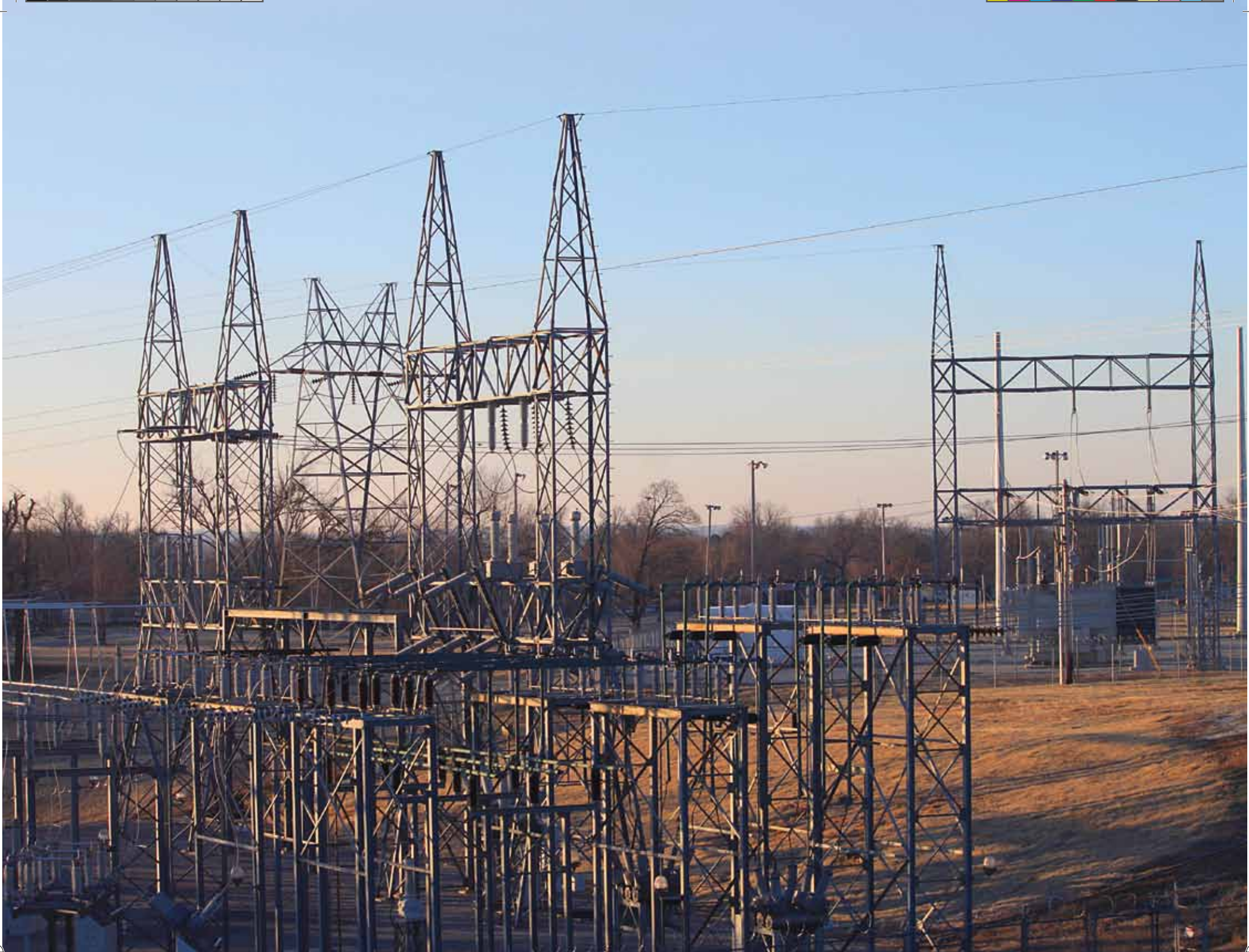
PENSACOLA DAM SUBSTATION
