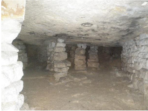
Figure 9. Example of an accessible ceiling supported by pillars, walls and filling backfill
