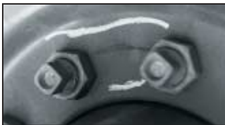
These cracks will continue to grow outward, through the "dish" or between stud holes.
