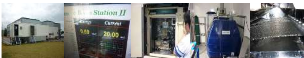
Fig.2. View of MEB installed in sewage treatment plant
