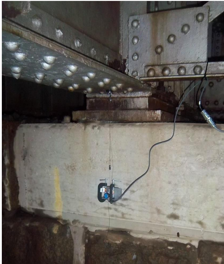
FIGURE 5.2 String potentiometer mounted near girder bearing.
