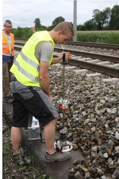
Figure 20: A LFW being used on an asphalt trackbed layer in Austria. (ÖBB – Austrian Federal Railway)
